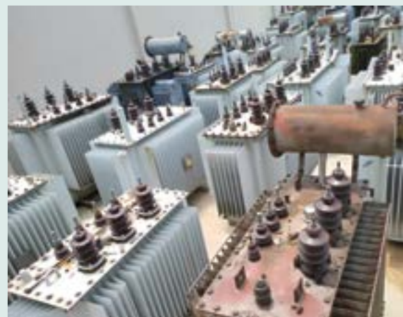
Storage of End-of-Life Power Equipment in Tongling, Anhui Province
